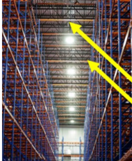
Overhead Rack Ties
